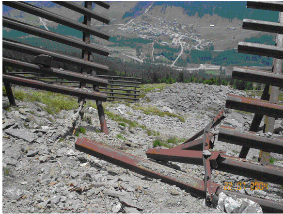
Fig. 9: Supporting structure damaged by rockfall.
