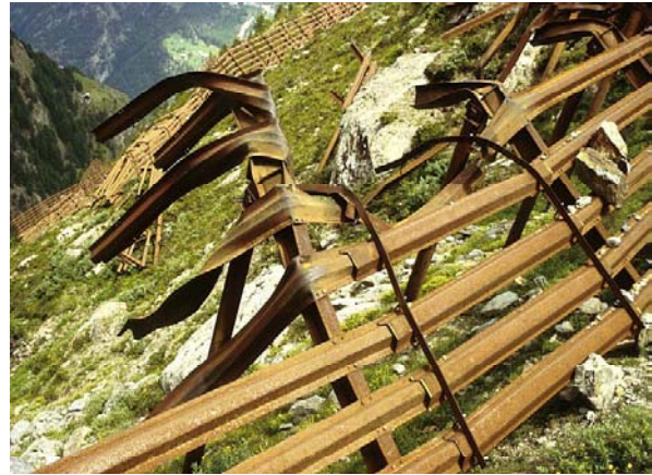
Fig. 10: Supporting structure damaged by avalanche impact.
